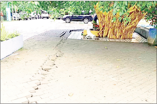
A view of the pedestrian platform and square near Strand Road on the Pathein Riverside, part of which the Ngawun River damaged.
